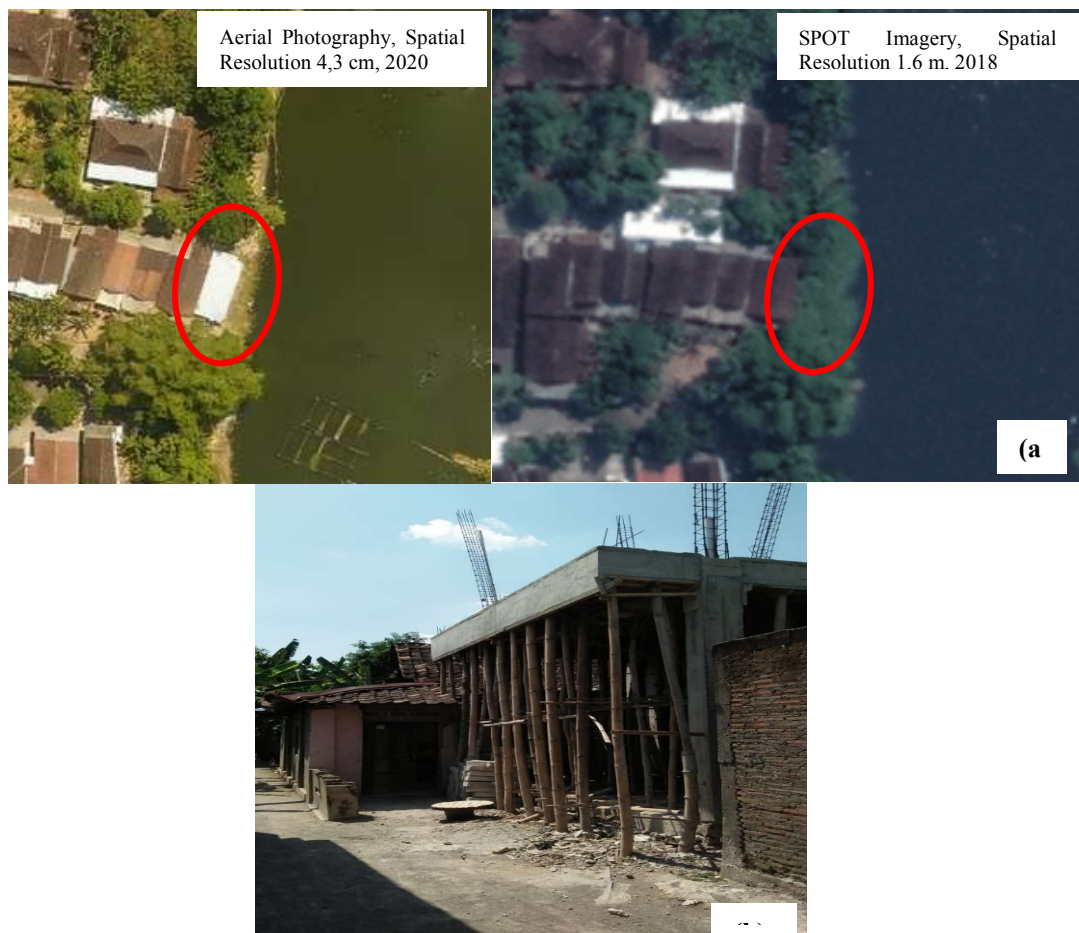
Figure 1. Landuse change: (a) Comparison Additional buildings seen from the SPOT imagery (2018) and Aerial Photography (2020); and (b) The construction is carried out around
