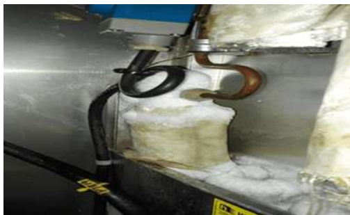
Figure 6 Exp. valve is blocked by ice
