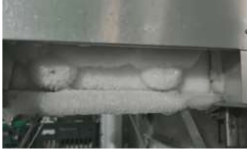
Figure 5 Evaporator is blocked by ice
