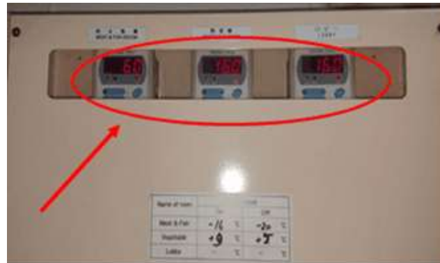
Figure 3. The cold room temperature panel has increased in temperature
