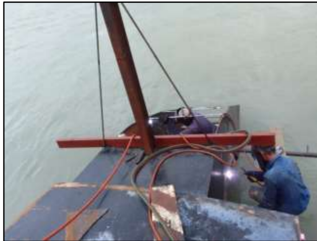
Figure 3. Tailing Chute Welding Work When the Weather Is Good Source: Personal Documentation (2022)
