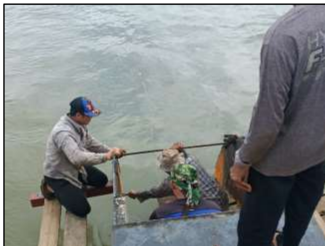
Figure 2. The process of replacing a 4mm Steel Plate and a 6mm Steel Plate Source: Personal Documentation (2022)
