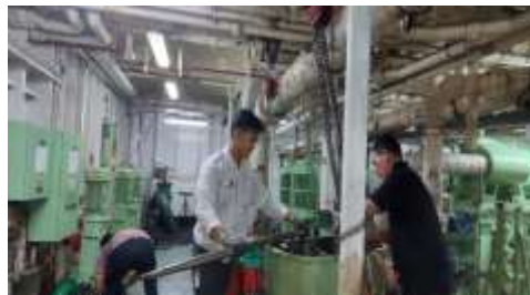
Figure 3. Machine crews work without using safety equipment
