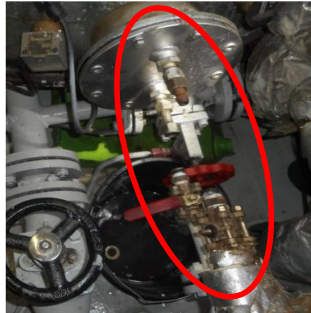
Figure 4. Steam valve inlet heater sludge tank Source: Private document, 2022
